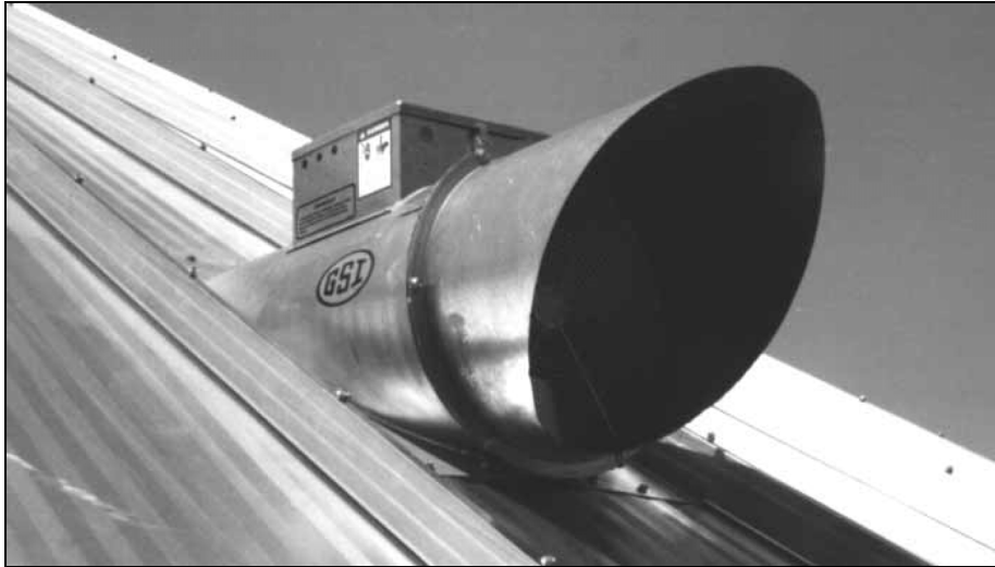
Figure 3A An 18" Roof Exhaust Fan
